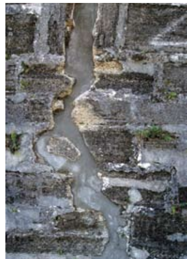
Crack in Castillo Wall
