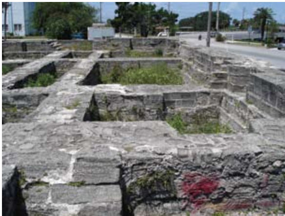
This is a photo of the New Smyrna coquina foundation, left over from the Turnbull Colony. Can you see all of the plants growing in it?
